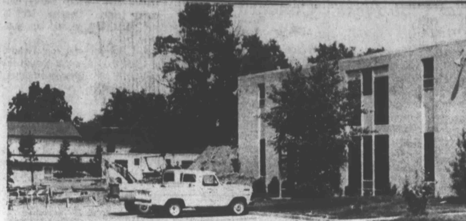
DIRT MOVING STARTED last week to enlarge the reservoir and filtering system at the Halls water plant. The Halls system has recently started serving 250 new customers in Unionville and Forked Deer communities.
